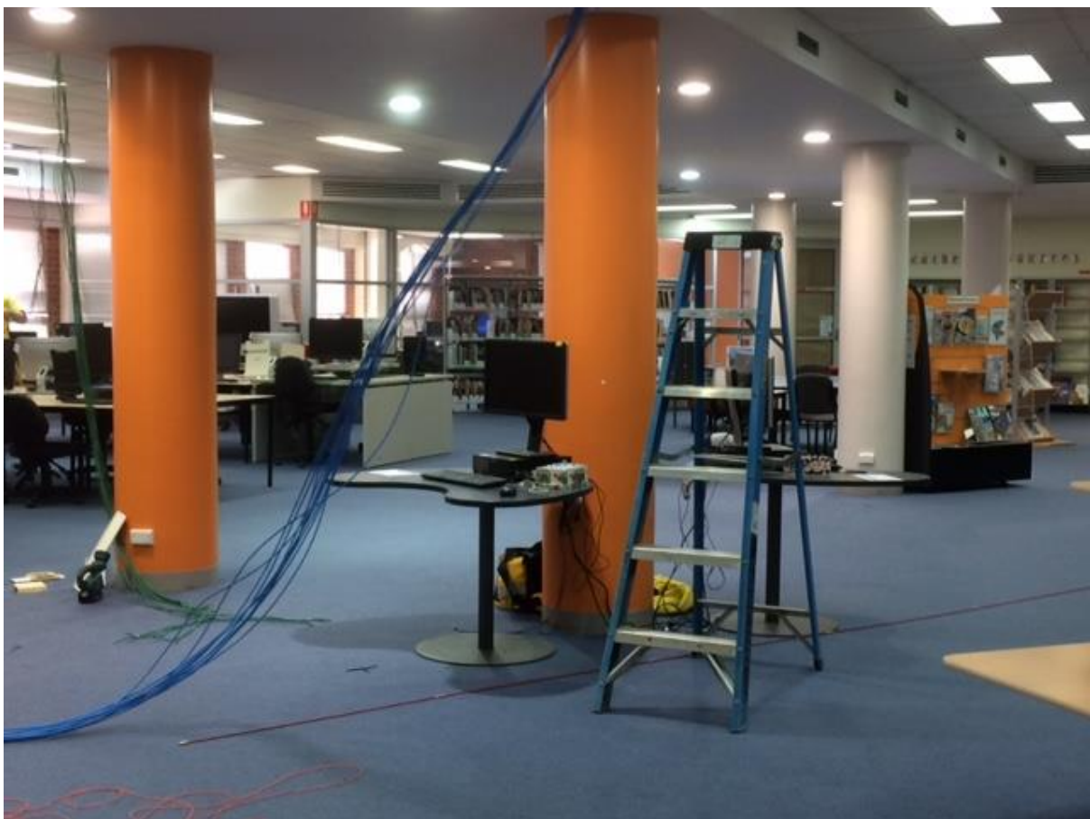
Cabling in Library while computers are moved
